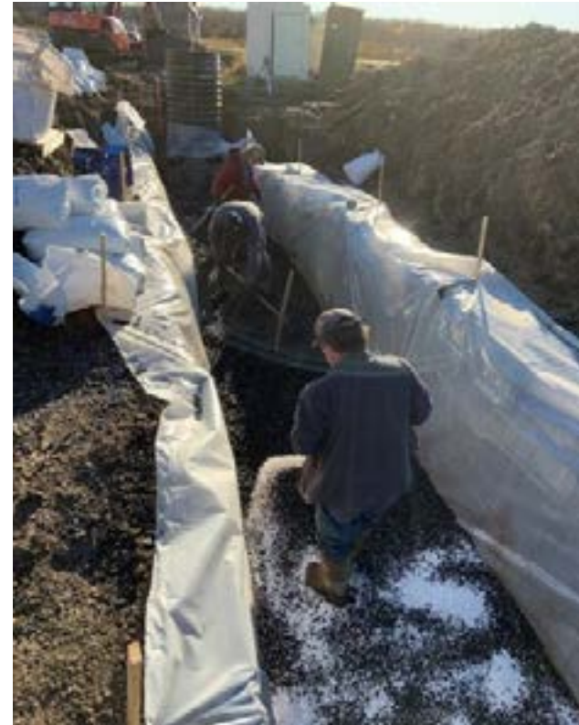
Constructing a P filter at the outlet of a tile drain in St. Albans
