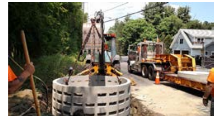
Image of a dry well getting installed on a previous Lake Champlain Basin Program funded project in the Town of Lake George. The Town of Lake George Highway Department installed the structure.
