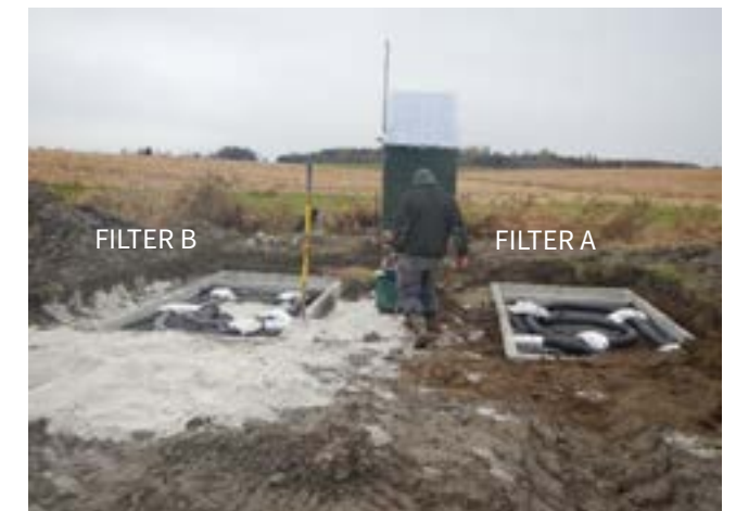
Phosphorus filters filled with media, prior to placing on lids. Filter B (left) was comprised of limestone “bedding sand” and Filter A (right) contained drinking water treatment residuals.
