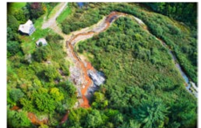
Aerial Photo of the Bogue Branch in the area of the removal of Johnsons Mill Dam. Credit Dana Allen of FluidState Consulting - September 21, 2021.
