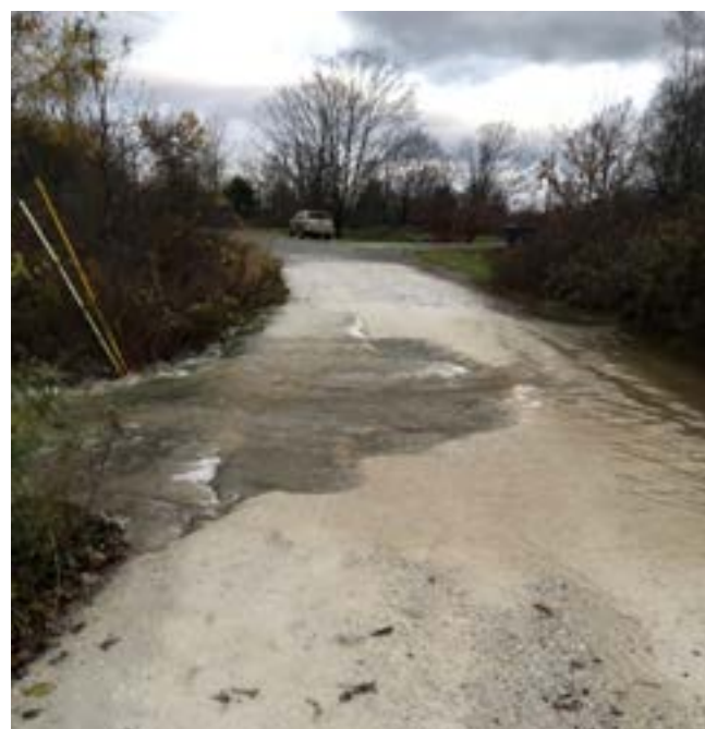
Neighborhood outreach to areas like this (where undersized culverts cause road washouts during flood events) will help citizens understand the importance of making fixes to improve downstream water quality. Photo credit Kate Kelly
