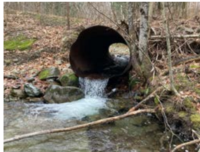
Undersized, perched culvert on private maple sugaring land in the Missisquoi River basin (Bakersfield, VT).
