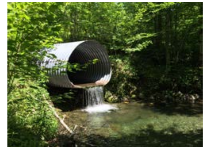
Purchase Brook culvert with roughly 2' drop to water surface at outlet and high levels of scour downstream of the culvert.
