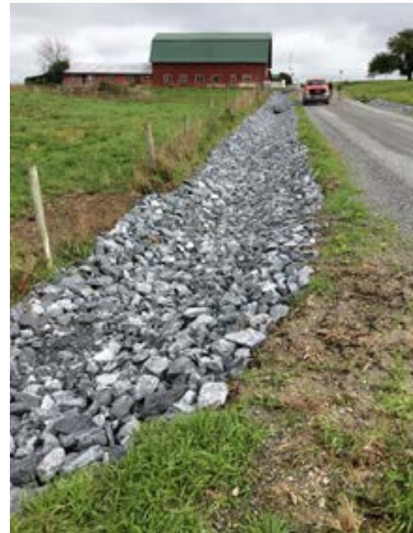
An example of a Best Management Practice (BMP) installed on a municipal road through the Municipal Roads Grants-In-Aid program. This type of BMP may be installed as part of the work plan for this grant project.
