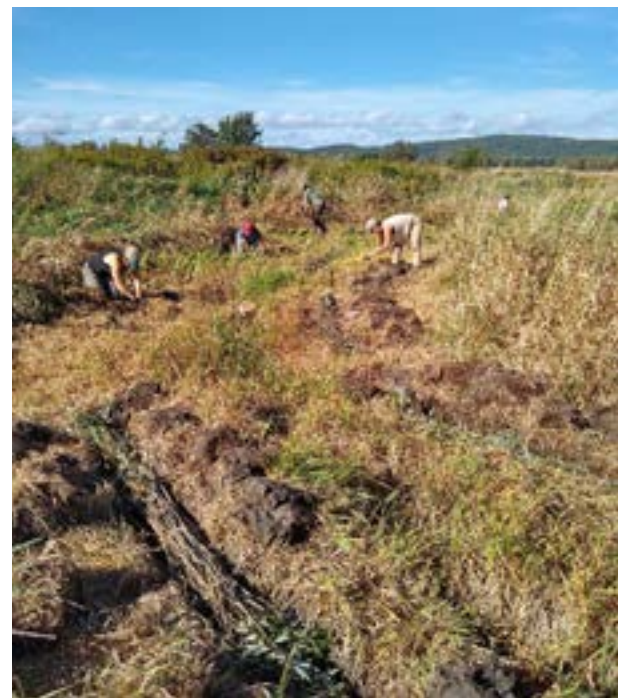
Fascine and live stake installation at a site in Cornwall in 2021. These areas had been prepped by clearing competing vegetation ahead of install, creating easier access, more efficient digging, better site conditions for establishment next season.
