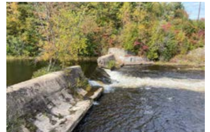
Indian Rapids Dam (44.67447,-73.49025) is an obsolete, breached, deteriorated concrete structure (Photo USFWS). The spillway that spans the river channel is 12 feet tall, 18 feet wide at the base, and 172 feet long (including the 55-foot breach). In addition to the removal of the spillway, a concrete/earthen powerhouse and platform will also be removed as part of the project. The dam is owned by New York State Electric and Gas (NYSEG).
