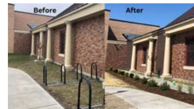
The northeast side of the Connector before and after building the infiltration trench and adding native shrubs to hold soil and reduce stormwater flows. The lawn did little to retain water during rain events and most of the stormwater would runoff into the adjacent sidewalk and parking lot. With the infiltration trench and planting, stormwater will have the chance to soak into the ground.
