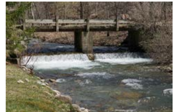
Sugar House Lane bridge sits atop a concrete structure that is a barrier to fish and other aquatic organism passage.
